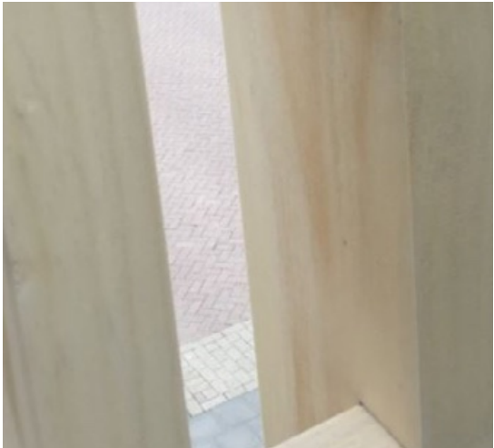
8.5 Reddish brown staining
